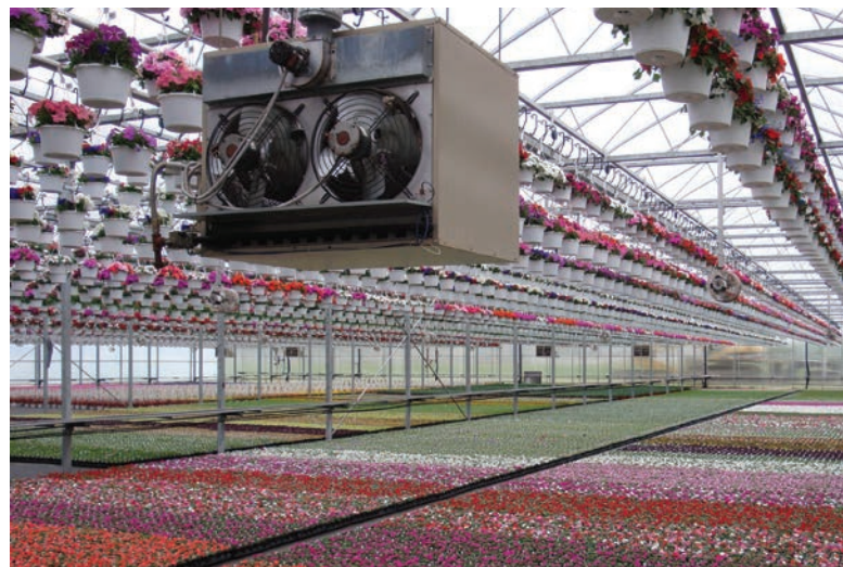
Figure 1. If growth of plants is stunted, flowering is delayed, or leaves start to twist or curl, ethylene contamination may be the problem. Check unit heaters to ensure adequate oxygen is provided for complete combustion of fuels, and that the exhaust is sufficiently ventilated.
